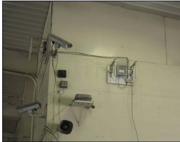
Figure 6: Low-voltage wiring and devices. Photo courtesy of Gladstein, Neandross & Associates, NREL
