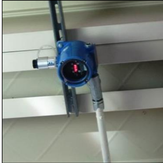
Figure 12: A ceiling-mounted combustible gas detection head. Photo courtesy of Sierra Monitor.
