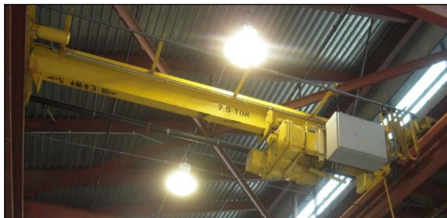
Figure 7: A typical overhead crane. Photo courtesy of Gladstein, Neandross & Associates, NREL
