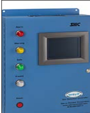
Figure 15: A combustible gas detection system control panel. Photo courtesy of Gladstein, Neandross & Associates, NREL
