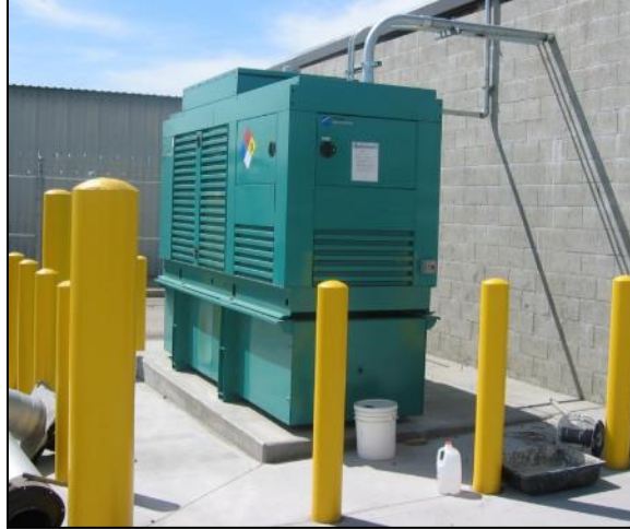
Figure 16: A typical emergency generator installation. Photo courtesy of Gladstein, Neandross & Associates, NREL
