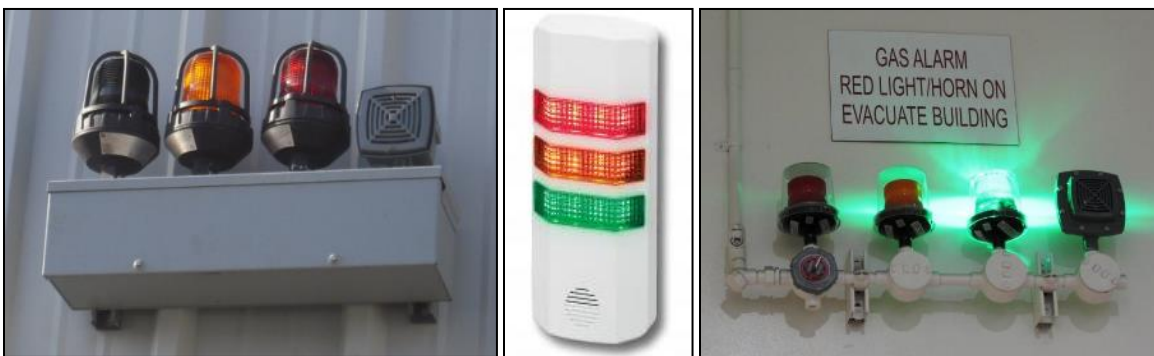
Figure 14: Examples of alarm status lights and horn panels (external and internal). Photo courtesy of Gladstein, Neandross & Associates, NREL
