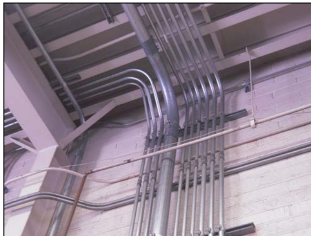
Figure 5: Relocating multiple conduits shown here would be costly and complex. Photo courtesy of Gladstein, Neandross & Associates, NREL
