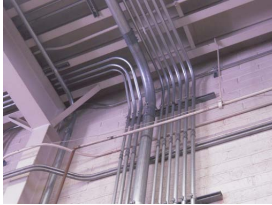
Figure 23: Relocating multiple conduits, such as those shown here, would be costly and complex. Photo courtesy of Gladstein, Neandross & Associates, NREL
