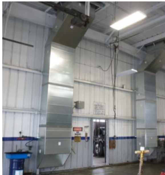
Figure 18: Conventional fuel maintenance facility ventilation pickup points near the floor. Photo courtesy of Gladstein, Neandross & Associates, NREL
