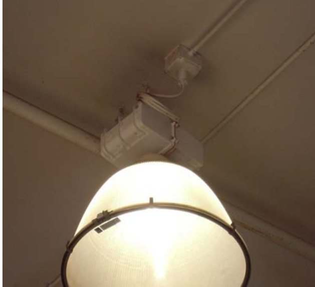
Figure 25: Overhead lighting fixture and ballast that are not yet lowered out of the classified zone. Photo courtesy of Gladstein, Neandross & Associates, NREL
