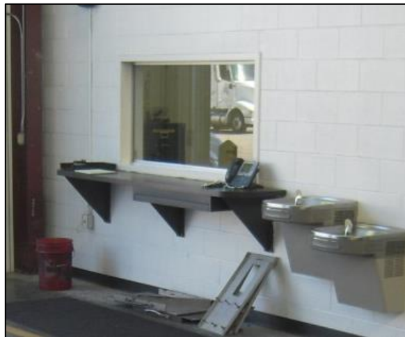
Figure 35: A pass-through window presents a potential path of migration. Photo courtesy of Gladstein, Neandross & Associates, NREL
