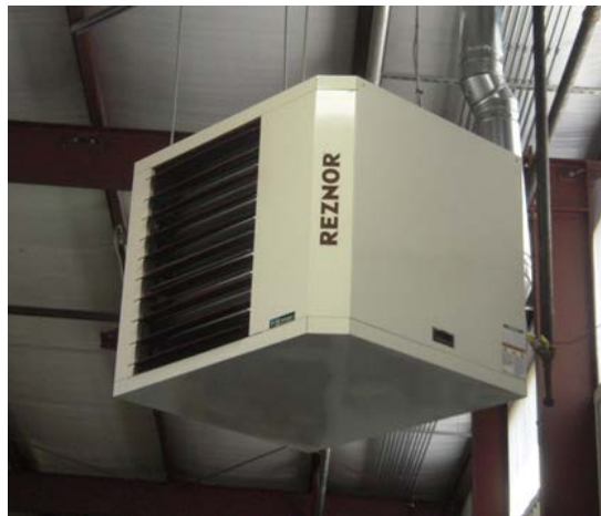
Figure 22: Ceiling-mounted gas-fired fan heater. Internal surfaces may be exposed and may present an ignition potential. Photo courtesy of Gladstein, Neandross & Associates, NREL
