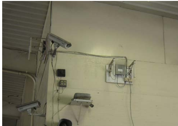
Figure 24: Low-voltage wiring and devices. Photo courtesy of Gladstein, Neandross & Associates, NREL
