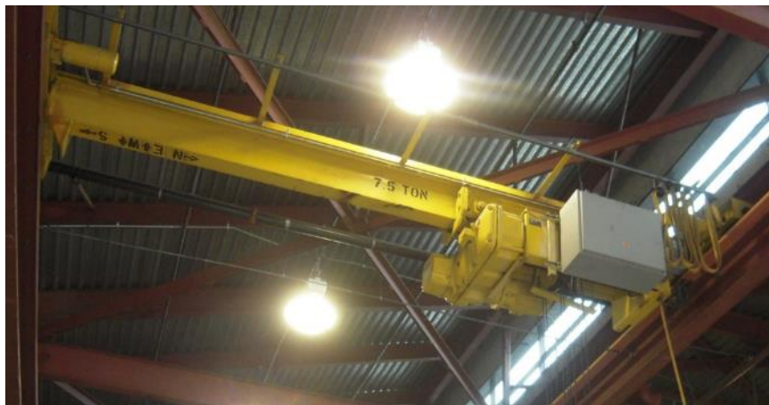
Figure 28: A typical overhead crane. Photo courtesy of Gladstein, Neandross & Associates, NREL
