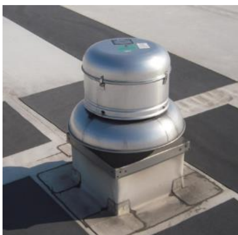
Figure 12: Roof-mounted up-blast fan. Photo courtesy of Gladstein, Neandross & Associates, NREL
