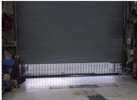
Figure 9: Security mesh in overhead doors. Photo courtesy of Gladstein, Neandross & Associates, NREL
