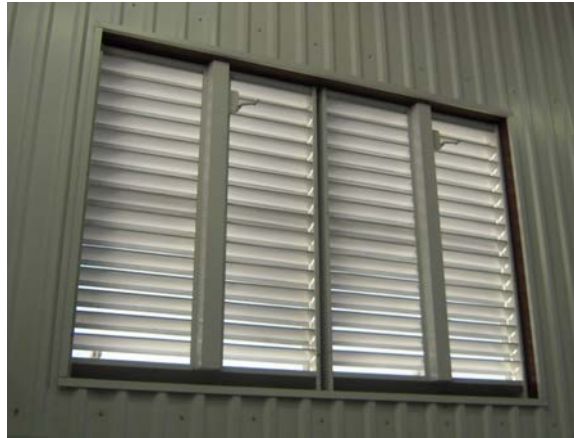
Figure 10: In-wall louver that provides makeup air flow. Photo courtesy of Gladstein, Neandross & Associates, NREL
