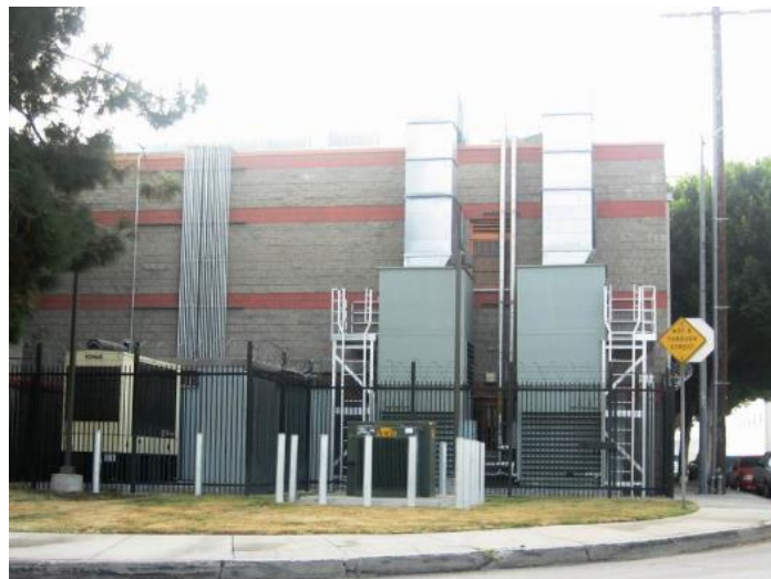
Figure 16: Ground-mounted fan with external ducting. Photo courtesy of Gladstein, Neandross & Associates, NREL
