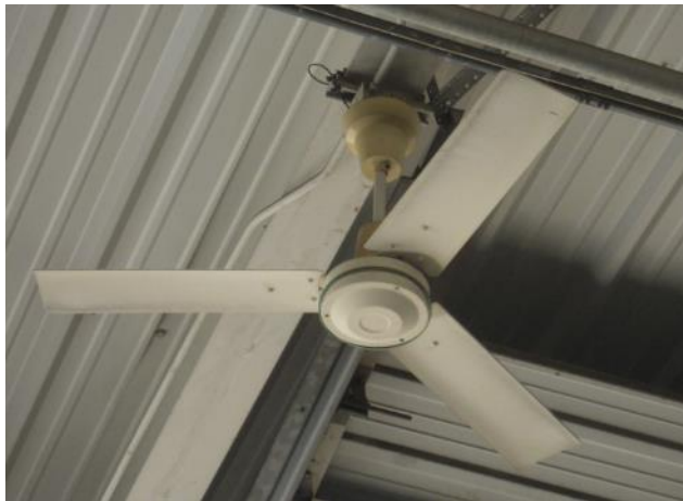
Figure 26: An overhead rotary fan that presents a potential ignition source. Photo courtesy of Gladstein, Neandross & Associates, NREL
