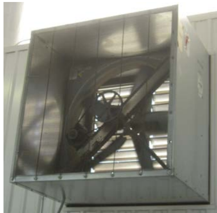
Figure 11: Powered sidewall fan that provides makeup air flow. Photo courtesy of Gladstein, Neandross & Associates, NREL
