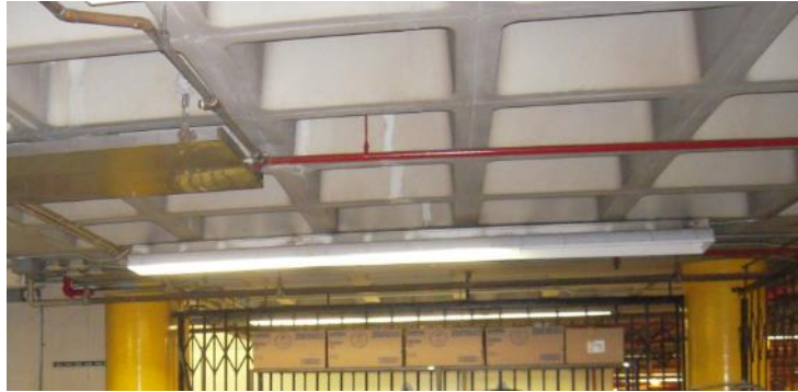
Figure 17: Ceiling configuration with “pockets”. Photo courtesy of Gladstein, Neandross & Associates, NREL
