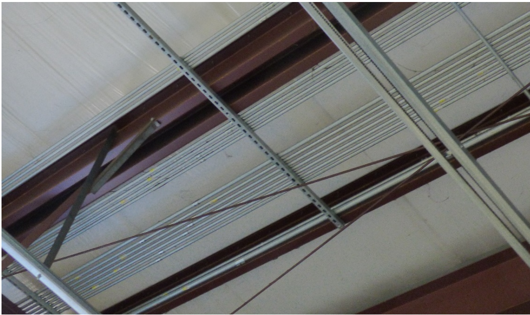
Figure 36: This conduit is within 18 inches of the ceiling. This is acceptable if the conduit is sealed against gas migration, but may need to be moved if it is a path of gas migration.
