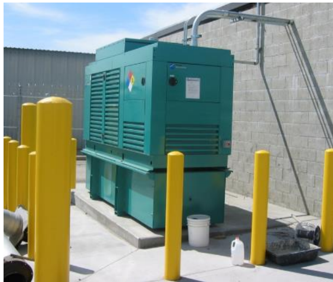
Figure 8: A typical emergency generator installation. Photo courtesy of Gladstein, Neandross & Associates, NREL
