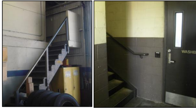
Figure 34: Stairways to upper levels are a potential path of migration. Photo courtesy of Gladstein, Neandross & Associates, NREL
