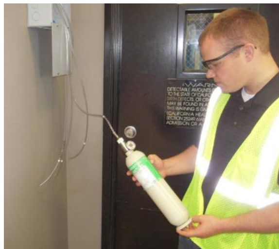
Figure 5: Gas detector calibration tubing. Photo courtesy of Gladstein, Neandross & Associates, NREL
