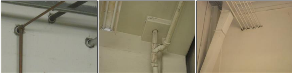
Figure 29: Unsealed conduit or pipes passing through walls or ceilings present a potential path of migration. Photo courtesy of Gladstein, Neandross & Associates, NREL
