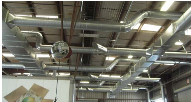
Figure 14: Ventilation ducting used to evacuate air from specific areas. Photo courtesy of Gladstein, Neandross & Associates, NREL
