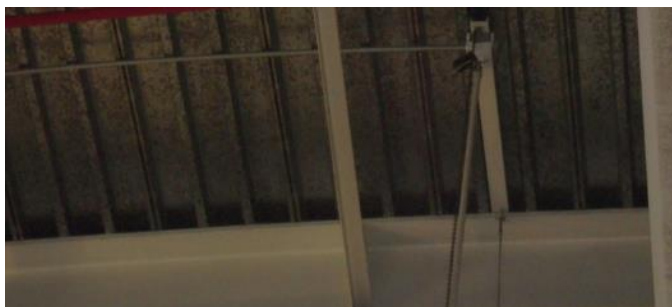
Figure 31: Gaps between walls and the ceiling present a potential path of migration. Photo courtesy of Gladstein, Neandross & Associates, NREL
